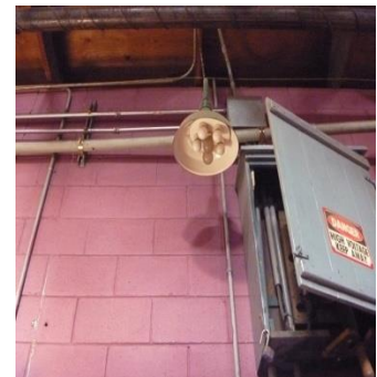
D/C Power Knife Switch Cabinet
