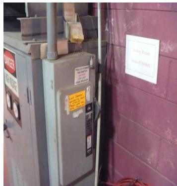
D/C Power Breaker
