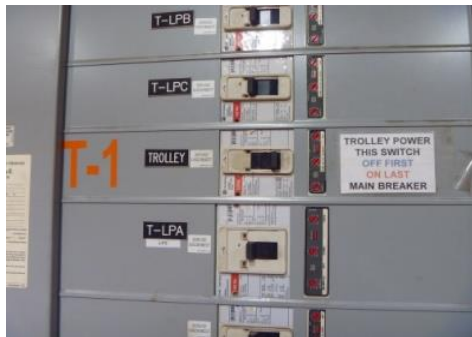
A/C Power Circuit Breaker
