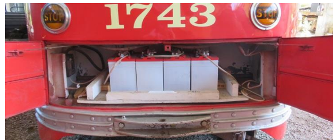
Battery Compartment with Both Doors Open. Battery Switch on Left Side of Compartment
